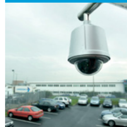
SPD-3300 dome in a fully weatherproof housing gives flexible viewing over the car park and building perimeter
