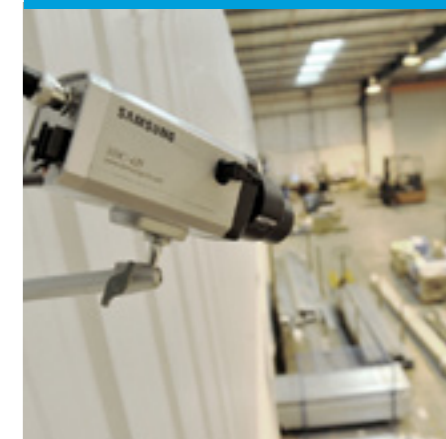
SDC-425 camera with wide-angle lens provides a full overview of the dispatch bay
