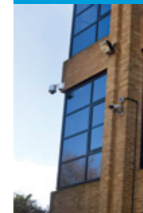
A mix of Samsung Techwin speed domes and static cameras protect the building's exterior.
