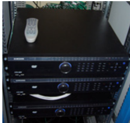
Just Three SVR-3200 DVRs record and control the entire installation
